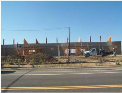
The Woodland Community College under construction on E Street near Husted Road.
